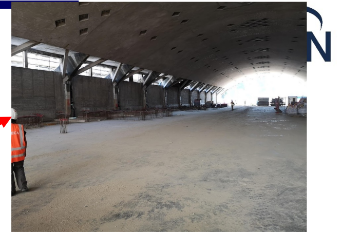
Each of the 6 “botti” (barrels) is ~5000m 2 of usable IT space
